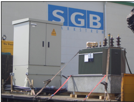
Spheres of competence of SBG Neumark: Transformers and compact-transformer-substations
