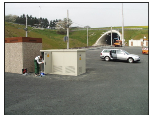
NDV401-train-transformer-substation with 16 2 / 3 Hz
