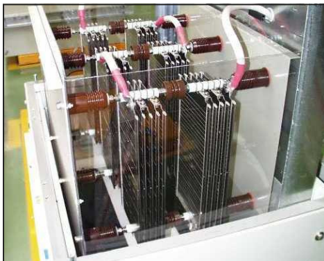
temporary low-resistance neutral earthing
